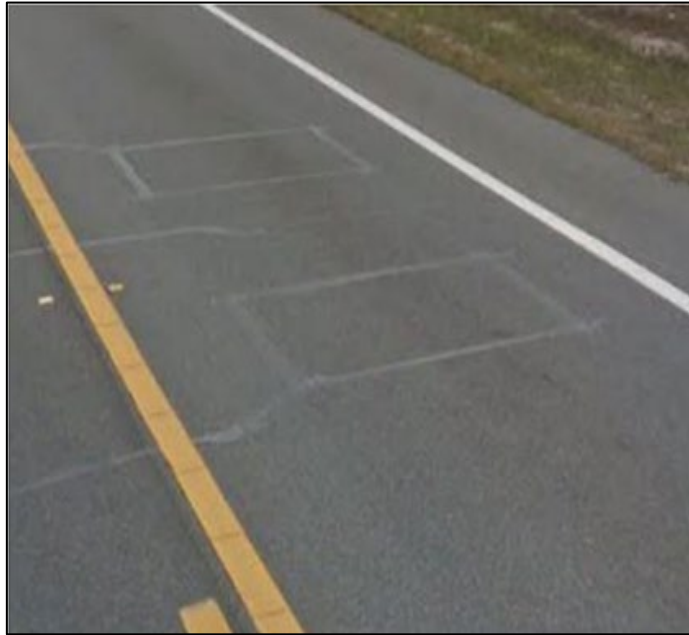
Traffic Monitoring System
