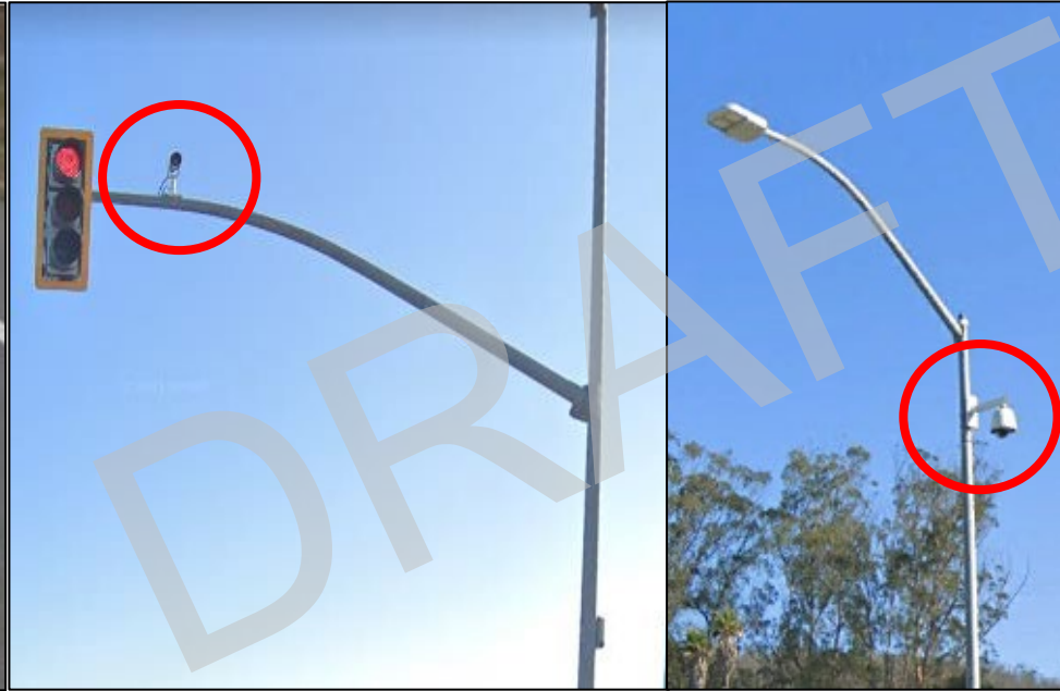
Fixed Intersection Camera/CCTV
