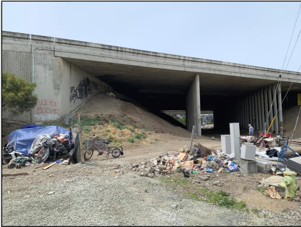
Photo 3. View southeast of Highway 101 underpass at east end of Segment 1 staging area.
