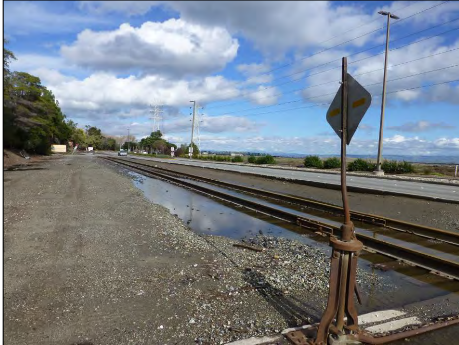
Photograph 3: At-grade railroad track paralleling Seaport Boulevard at switch south of siding, camera facing north, December 16, 2014.
