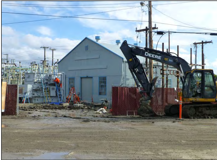
Photograph 2: North and west side of control house, camera facing southeast, December 16, 2014. Note installation of new transformer.
